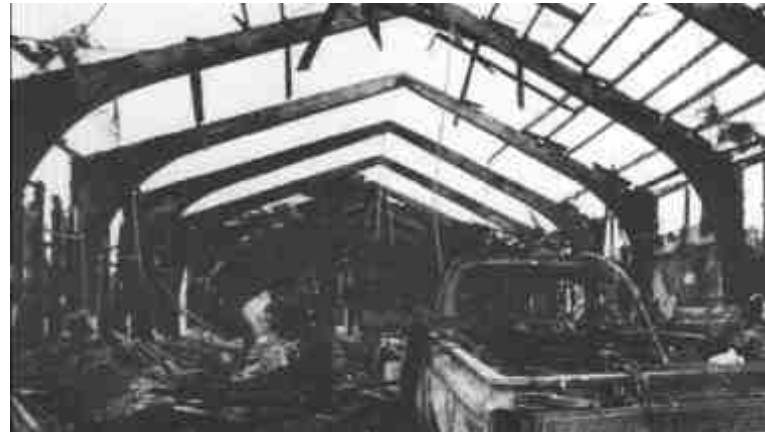
These Glulam portal frames maintained their integrity in a magnesium-fed fire. The metal walls and roof of the building melted and collapsed
